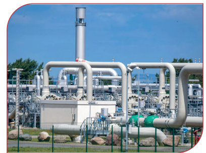
Gas Gathering Station Shahdol, Madhya Pradesh
