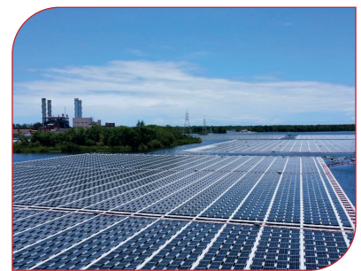
NTPC Floating Solar Power Plant Kayamkulam, Kerala
